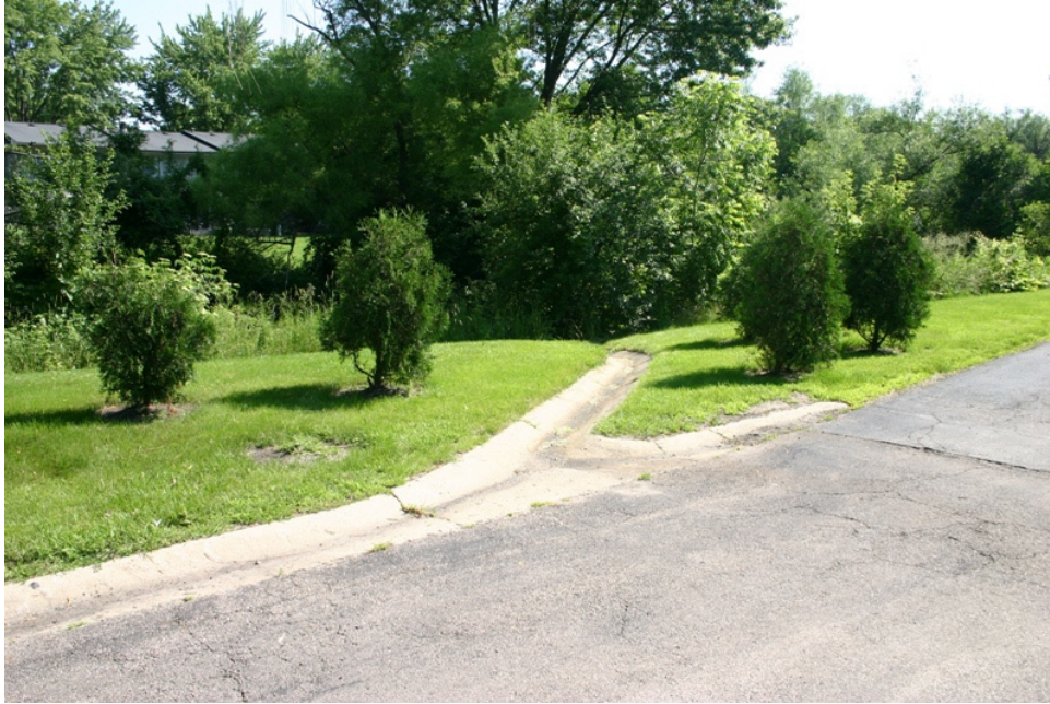
Above: Condominium parking lot runoff routed directly to Tyler Creek (Lower Tyler Creek Subwatershed).
