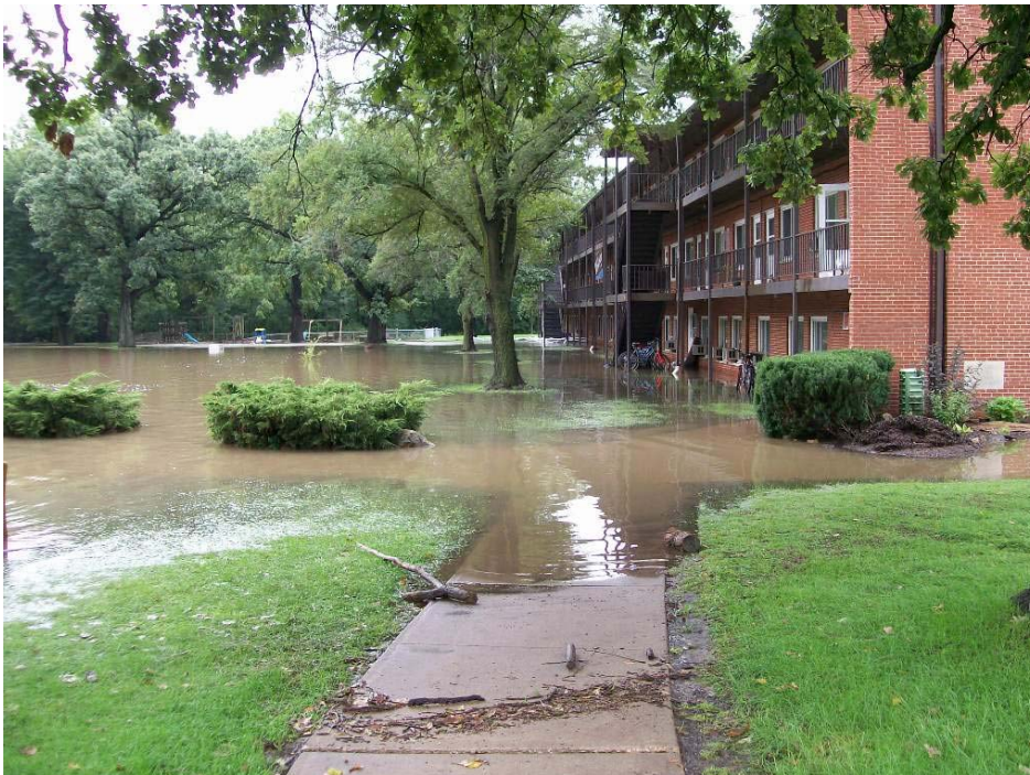
Right: Photo of flood damage to building on west side of Judson University campus following a August 2007 thunderstorm
