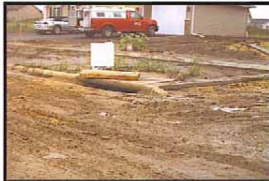
Fig. 13—No storm drain inlet protection
